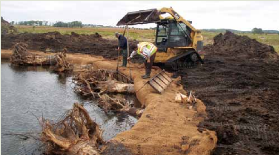
A TOE WOOD INSTALLATION ON THE VERMILLION RIVER, DEMONSTRATING SOME OF THE METHODS USED ON HAY CREEK
