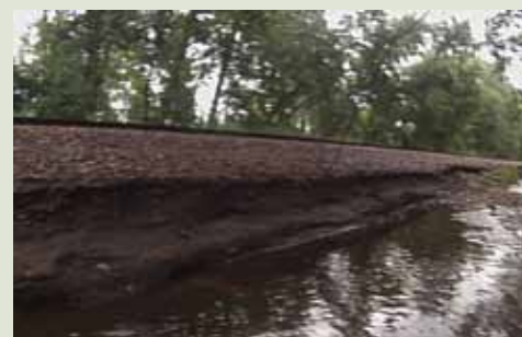
THE POTENTIAL UNNAMED #7, CEDARBRIDGE CREEK, FLOWING ALONG THE RAILROAD TRACKS AND CAUSING SIGNIFICANT DAMAGE AND EROSION.
