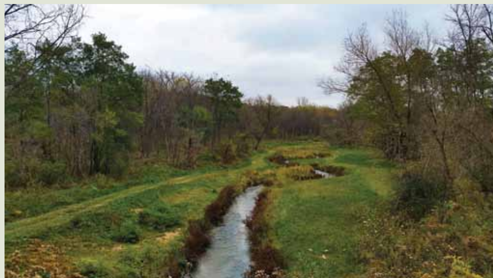
TOP: IT LOOKS NATURAL, BUT INVASIVE TREES AND ERODED BANKS MADE THE WATER WIDE, SHALLOW, SILTY AND DEVOID OF GOOD AQUATIC HABITAT. MIDDLE AND BOTTOM: MAJOR RESHAPING OF BANKS AND NARROWING THE CHANNEL DEEPENS THE STREAM TO FLUSH OUT SEDIMENT AND RESTORE GRAVEL BOTTOM. THE PROJECTS LOOK ROUGH FOR A FEW DAYS, BUT WITHIN WEEKS, THE RESTORATION WORK IS STABILIZED, AND THE BENEFITS WILL LAST FOR YEARS.
