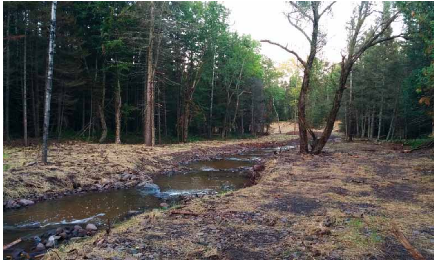
LITTLE STEWART RIVER - AFTER: OUR PROJECT RESTORED A STABLE CHANNEL WITH A SERIES OF DEEP STEP POOLS. THE FLOODPLAIN WAS RESTORED TO QUICKLY DISSIPATE FUTURE FLOODS' ENERGY. NOTE THAT THE TREE ON THE RIGHT BANK OF THE STREAM IS THE SAME TREE IN THE PHOTO IN THE ABOVE LEFT.
