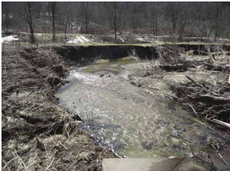
BEFORE: A TYPICAL ERODING STREAMBANK
